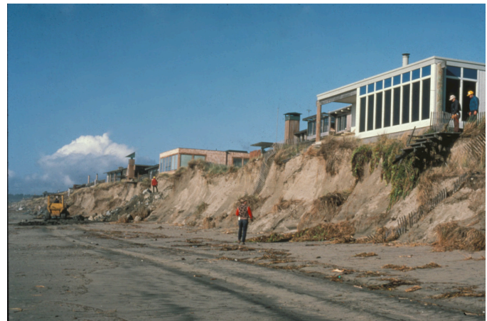
Figure 3.4. Dune erosion threatening homes in the Pajaro Dunes area of central Monterey Bay during the 1983 El Niño.
