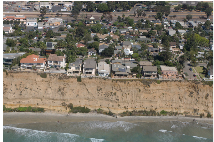
Figure 3.24. Lack of a fronting beach leads to continuous wave attack. A small rise in sea level will in all likelihood have a significant impact on cliff erosion in such areas (Kenneth and Gabrielle Adelman, California Coastal Records Project).
