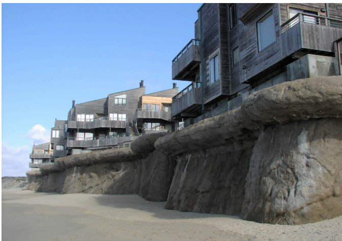
Figure 5.1. Ocean Harbor House condominiums in Monterey were built too close to an eroding dune face, which ultimately led to the construction of a massive concrete seawall for protection.
