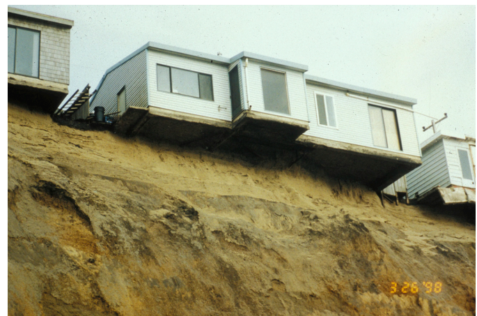
Figure 3.5. Bluff top homes in Pacifica, San Mateo County, were undermined and ultimately demolished during the 1997-98 El Niño.
